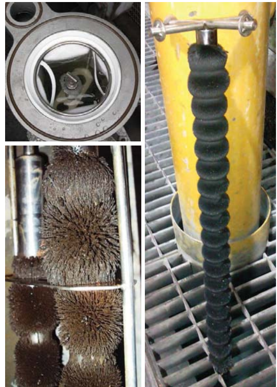
Top Left: Close up of saturated core. Bottom Left: Core tube assembly installed in P2 bag filter. Right: Standard P2 bag core tube saturated with ferrous material.
